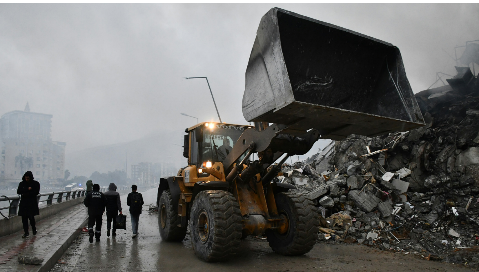
© Çağlar Oskay - İskenderun, Hatay Turkey - February 2023: In İskenderun, one of the places most affected by the 7.7 magnitude earthquake centered in Kahramanmaraş
